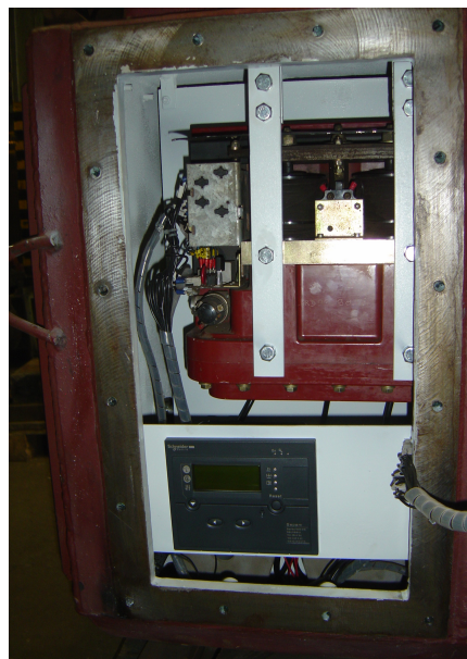
View of the GN chamber - side of the contactor
